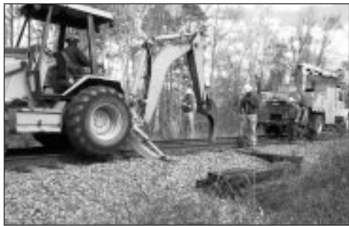
A test tie in the Cordele, Ga., test is being removed from the track for evaluation.
